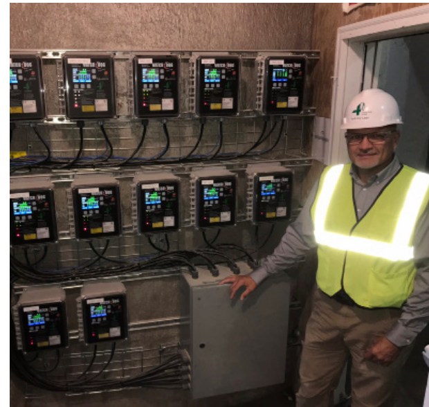
Several Watchdog Super Elite and Flex-Net Industrial Ethernet Systems installed in a facility control room
