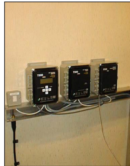
4B HotBus™ system installed in a facility control room
