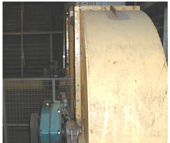
Main Intake Elevator
