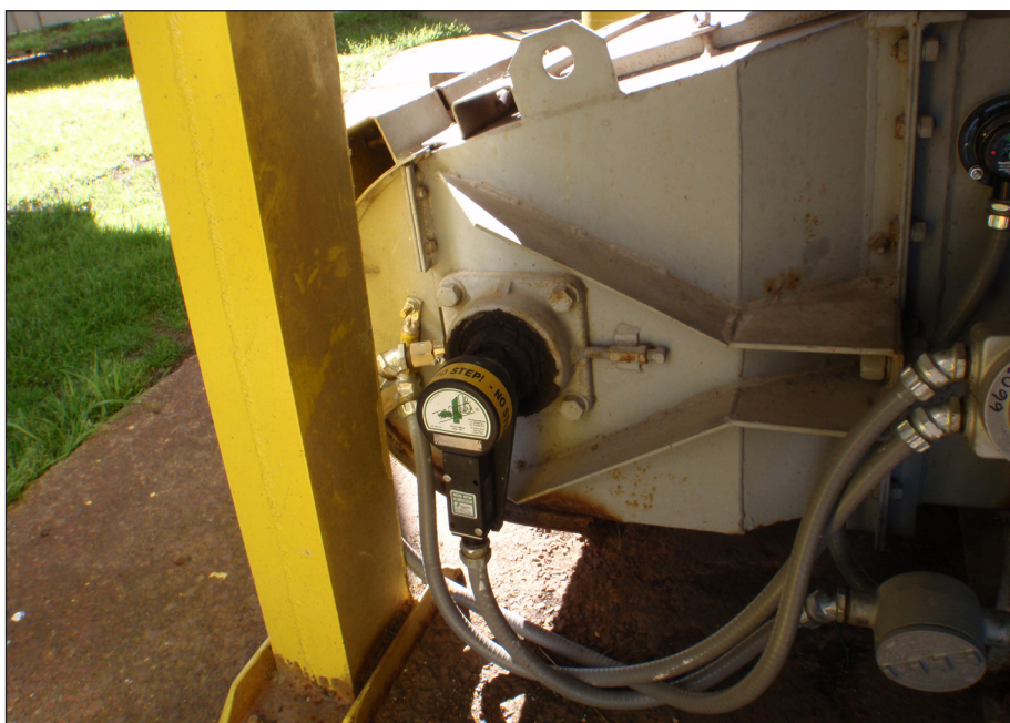
Whirligig® Installed on the Tail Shaft of Enclosed Conveyor with M800 Elite Speed Switch
