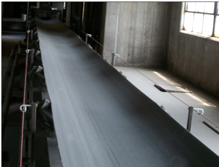
Pull Wire Installation with Pigtails Every 3m (10 ft.) at Grain Handling Facility
