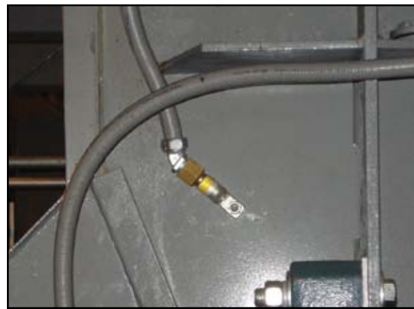
WDB70V3C lug style temperature sensor shown installed on enclosed belt conveyor casing.
