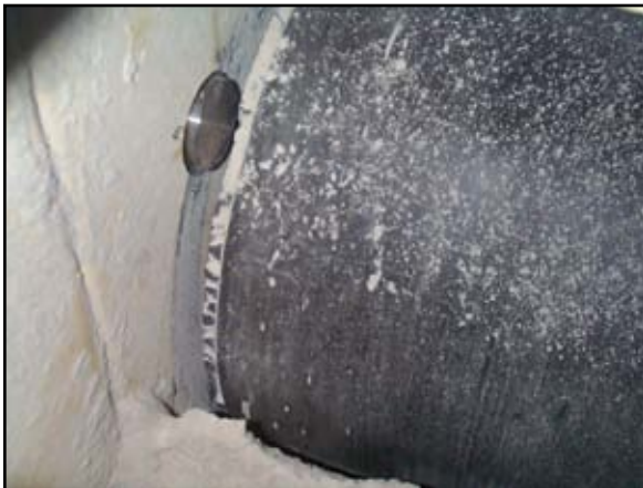
Touchswitch installed at the drive end of an enclosed belt conveyor (inside view).
