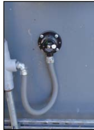
Touchswitch installed on a bucket elevator.
