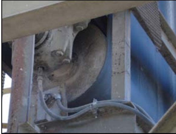
Touchswitch installed on take-up pulley of an open belt conveyor.
