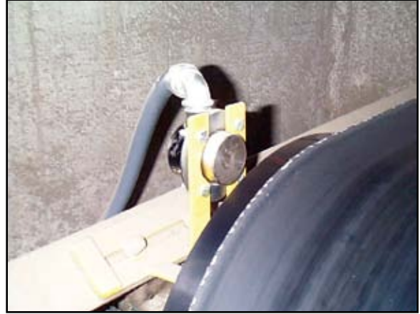
Touchswitch installed at the tail of an open belt conveyor.
