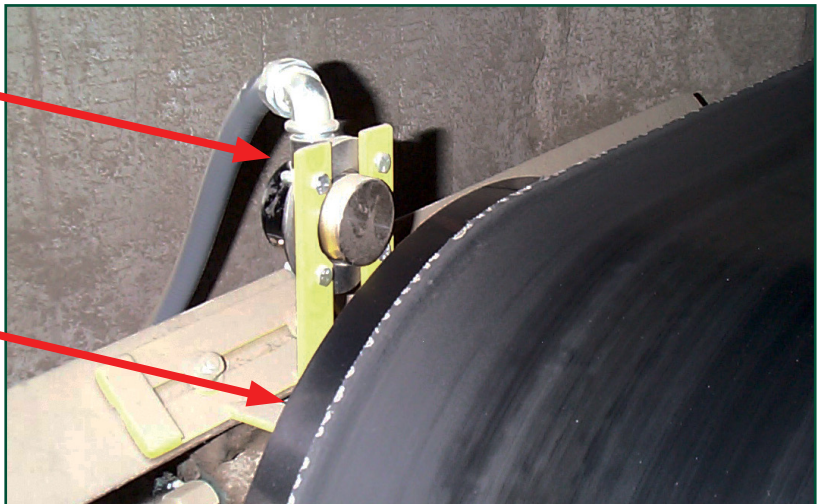
Touchswitch™ Installed at Tail of Open Belt Conveyor
