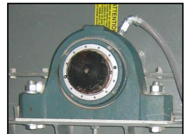
Bearing Sensor on Belt Conveyor
