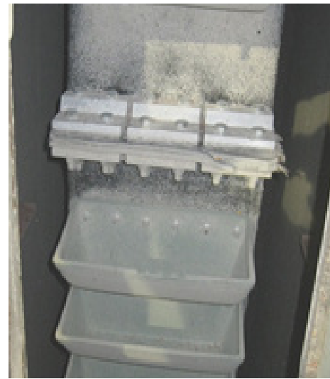
4B JUMBO™ CC-S® 16x8 low-profile buckets, 4B Braime Clamps & 1,000-piw rubber belting installed
