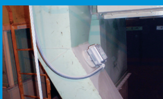
Auto-Set™ Flush Probe Installed on Belt Conveyor Discharge
